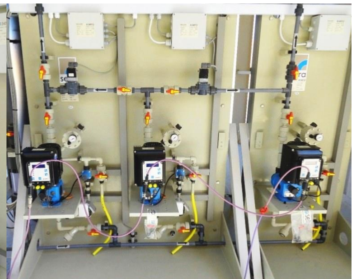
FeCl3 Dosing Unit (Front view)
