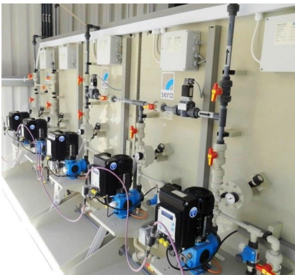
NaOH Dosing System (Side view)
