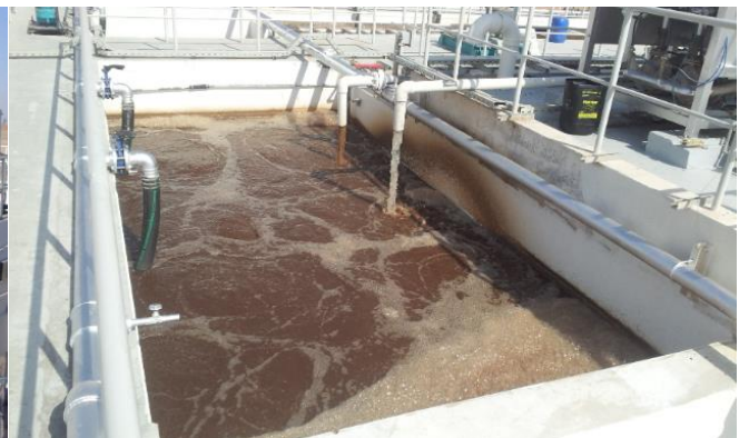
Membrane Bio Reactor
