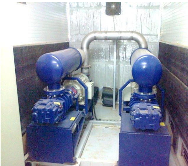
Air Blower for Aeration and MBR
