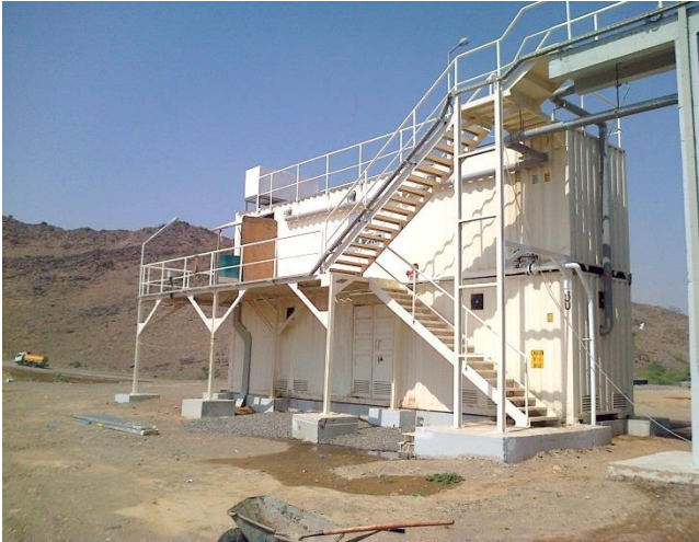
MBR Container Sewage Plant
