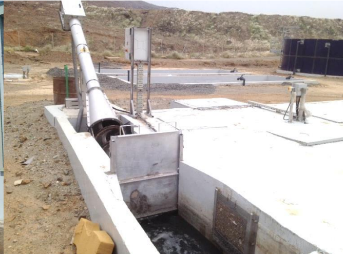
Screening Channel for Tanker Discharge
