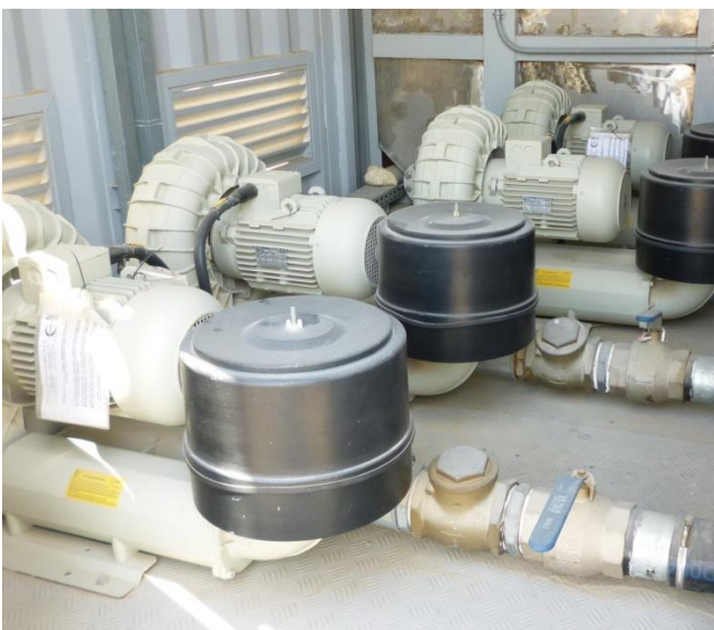
Air Blowers for Aeration and MBR Scouring
