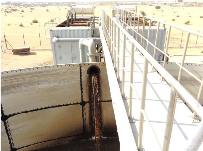
MBR Container Sewage Plant
