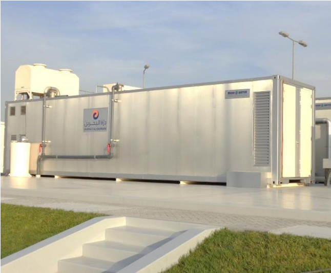
MBR Container Sewage Plant
