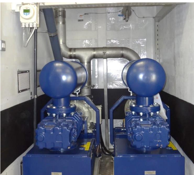
Air Blowers for Aeration and MBR Scouring
