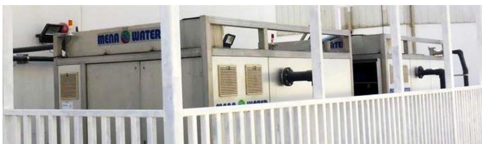
Sewage Plant with very small Footprint
