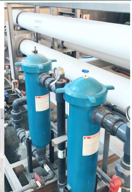
Reverse Osmosis Unit
