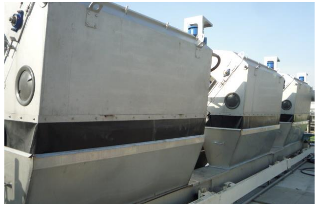
closed screenings discharge
