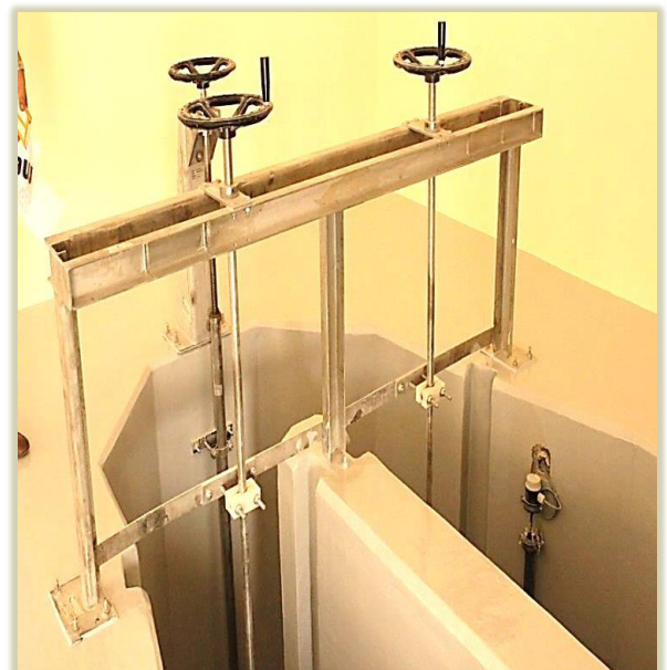
Penstocks with 3 Sides Ring
