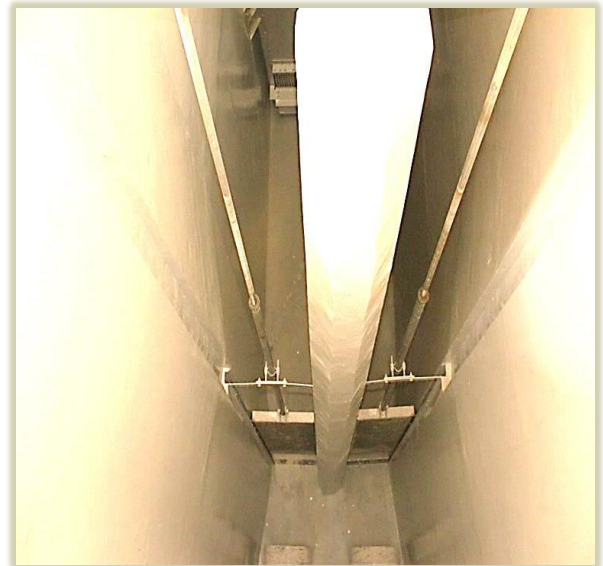
Penstocks with 3 Sides Ring
