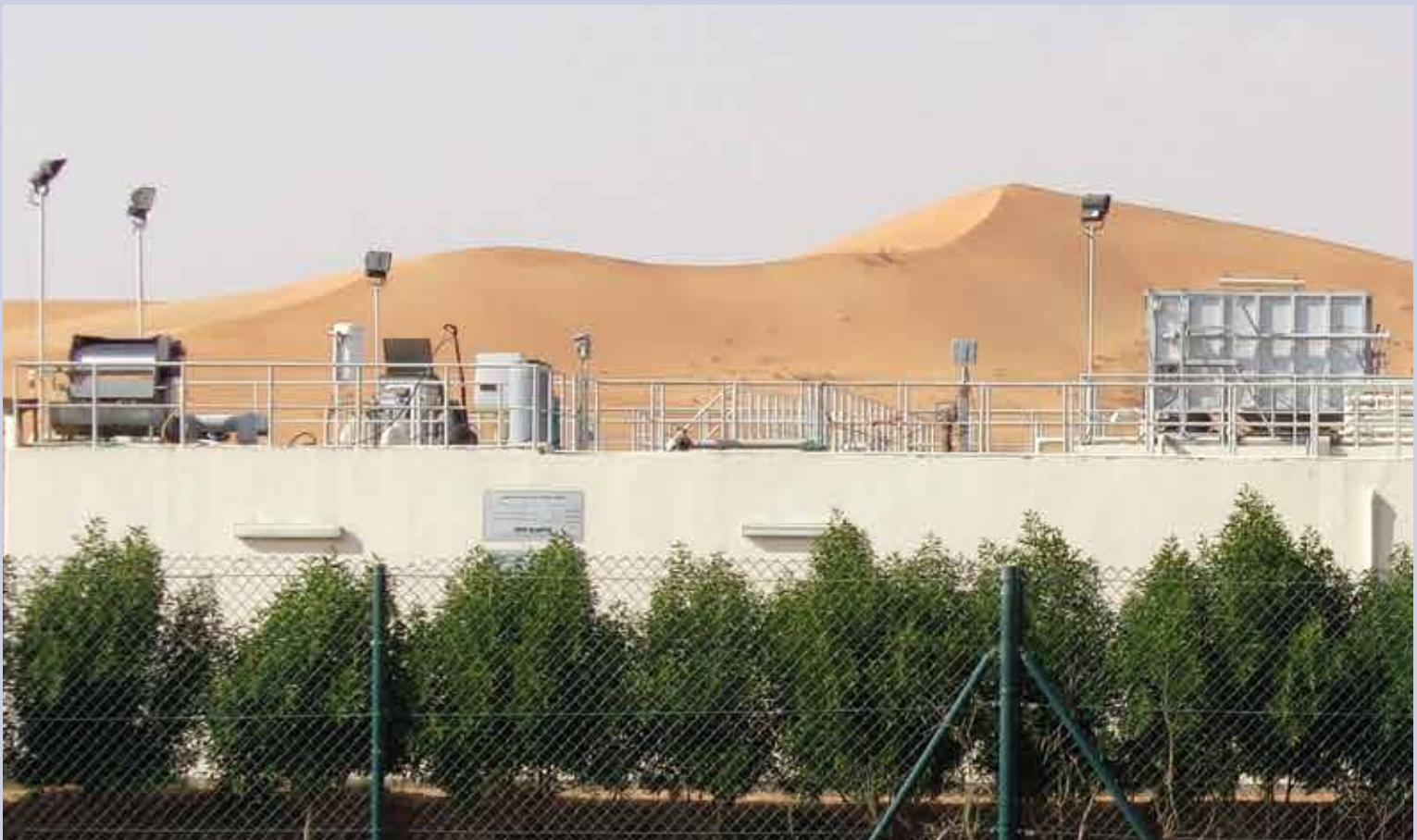
Al Ain Poultry Chicken Slaughtering & Processing, Effluent Treatment Plant, 400 m 3 /d Industrieabwasserreinigung, Al Saad, Al Ain – VAE
