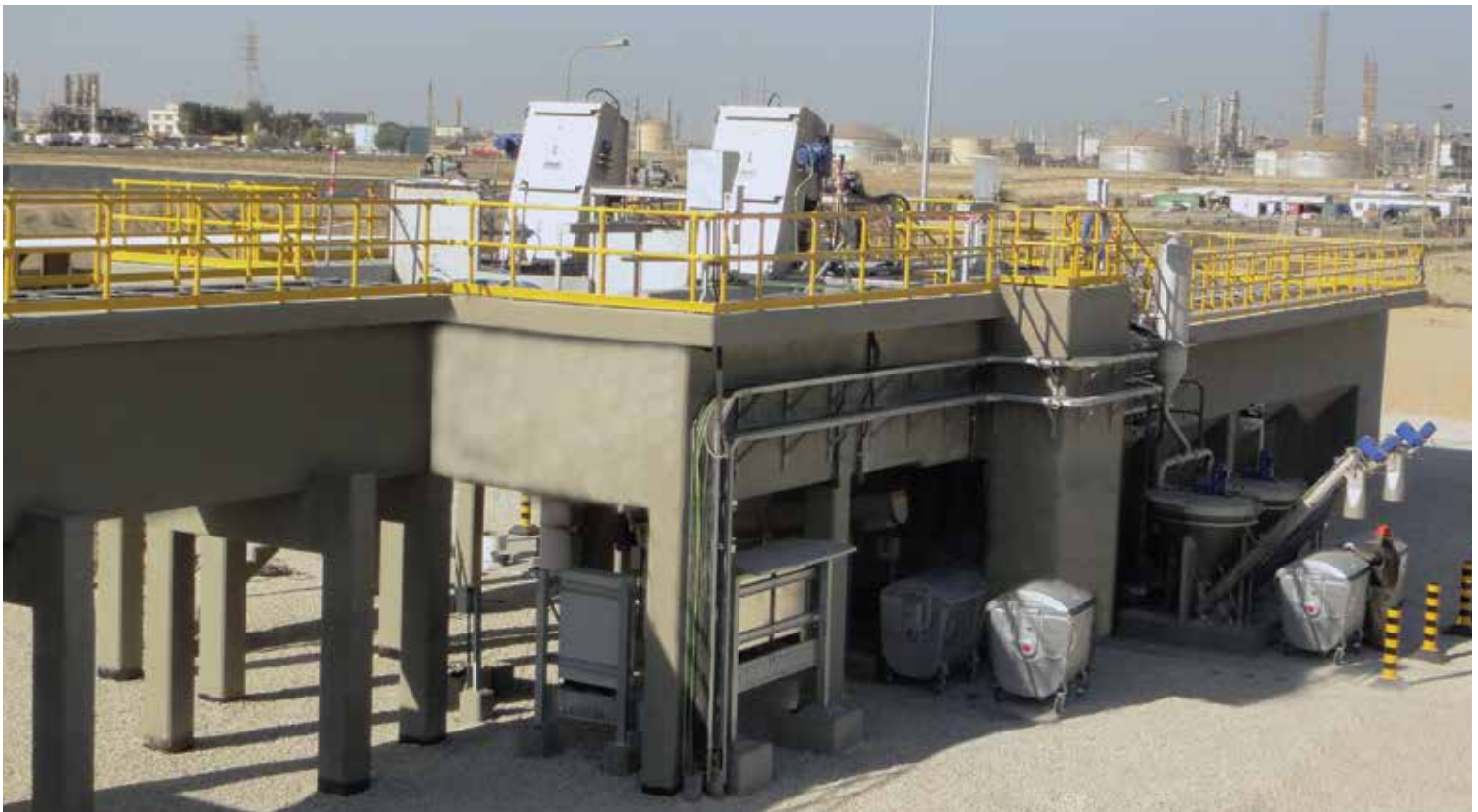
Marafiq Wastewater Treatment Plant, Pretreatment 66000 m 3 /day, Jubail - Saudi Arabia
