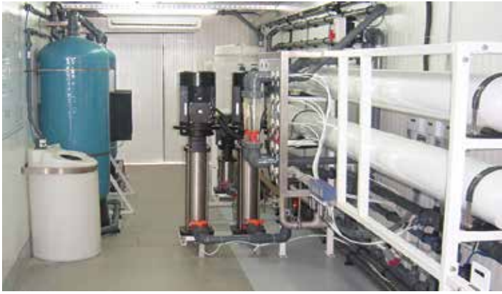
Station RO en conteneur - Al Mansuriya, Iraq
