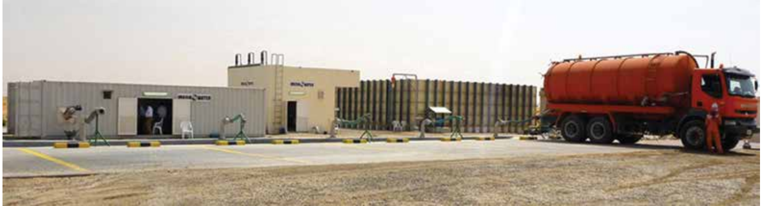
Bataya - station STP (MBR) - Sharjah, EAU
