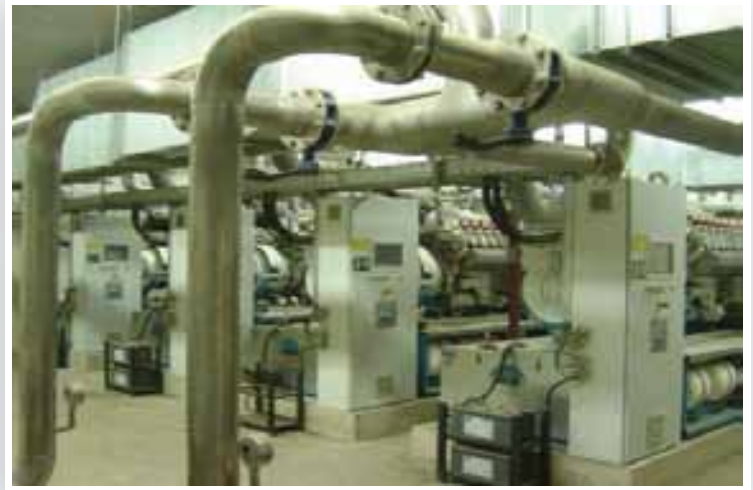
Co-generator - 1.3 MW – food waste
