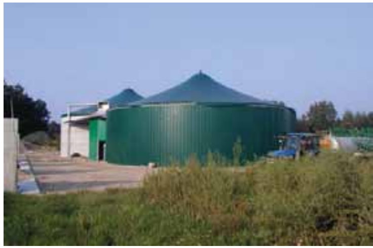
Biogas plant - 500 kW - manure and silage
