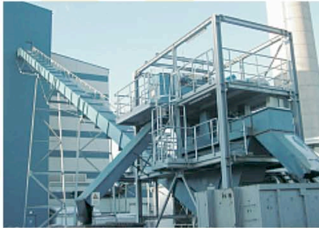
Enclosed belt conveyor and screening/separation at a re-cycled wood combustion plant.
