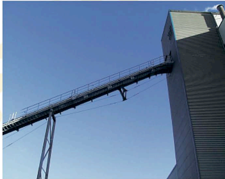
Conveying, storage and dosing of re-cycled wood
