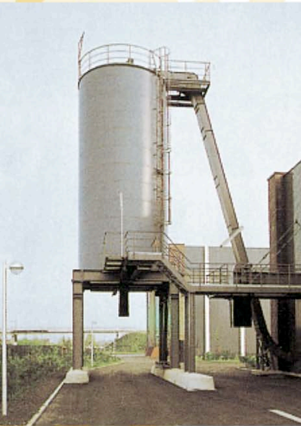
Truck loading silo for sludge cake
